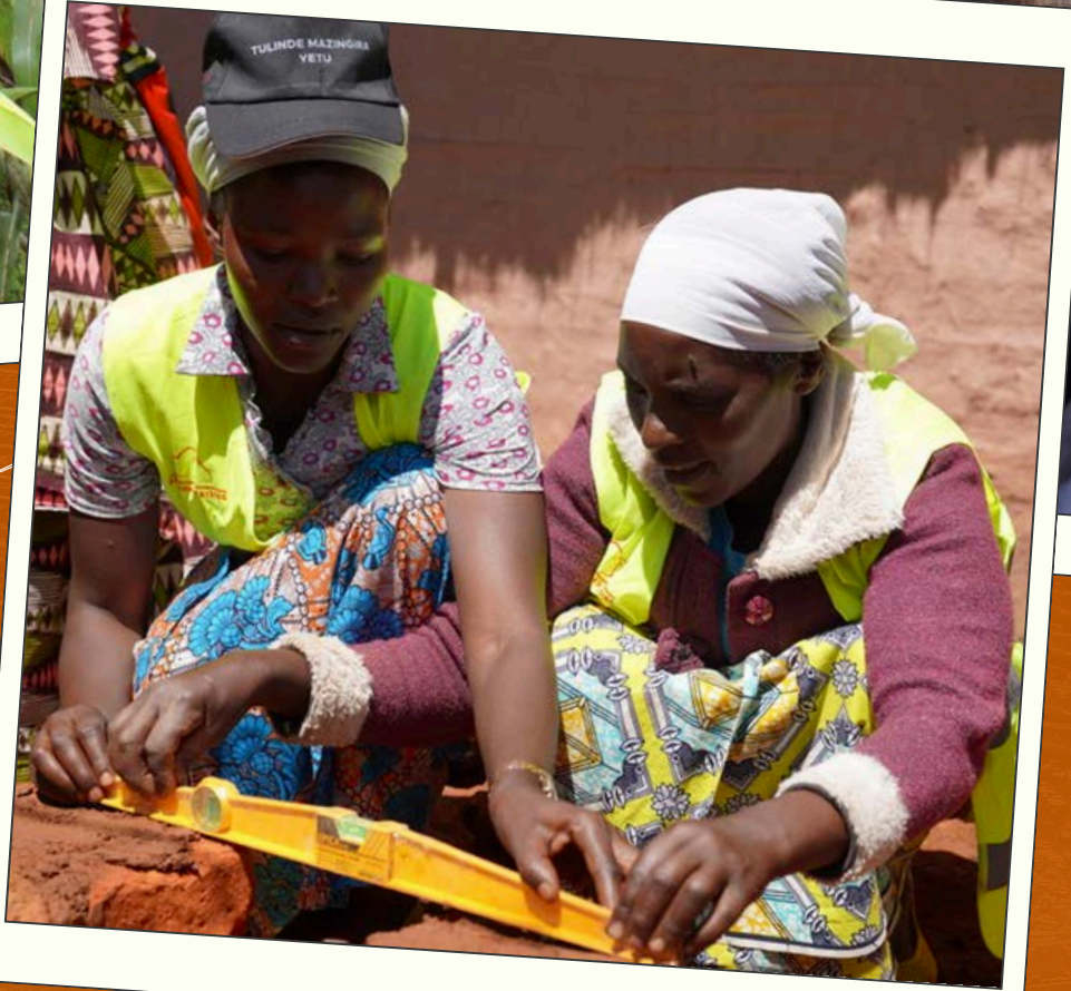
Women training to design and construct improved cookstoves to increase firewood efficiency and reduce deforestation pressure on the Itombwe Reserve.
